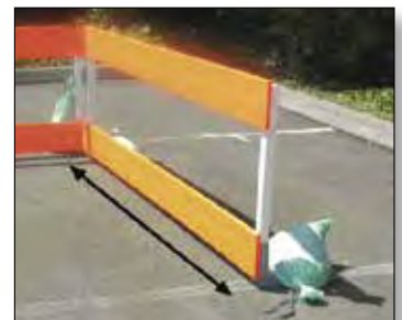
No part of the barricade protrudes into the walkway
